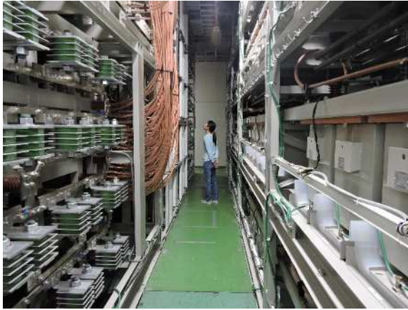
Huge Capacitor Bank System
