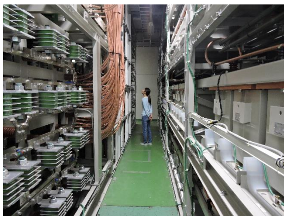
Huge Capacitor Bank System
