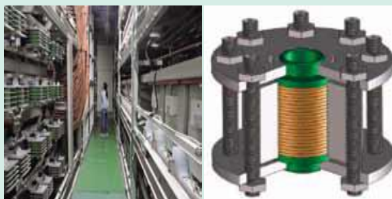
Huge capacitor bank system, and cut-view of a wide-bore pulse magnet
